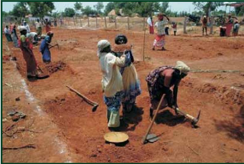
Rural Development : Workers laying road in Thirukannurpatii Village in Thanjavur District under the National Rural Employment Guarantee Act (NREGA). Photo : M. Srinath
